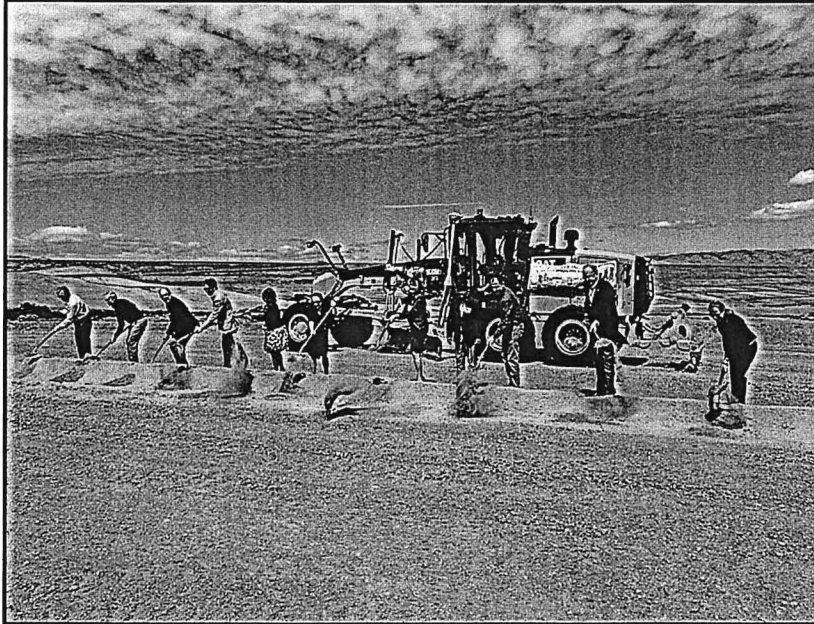
Dirt is turned on the B.F. Sisk Dam Safety Modification Project, June 17, 2022. Photo source: USBR
